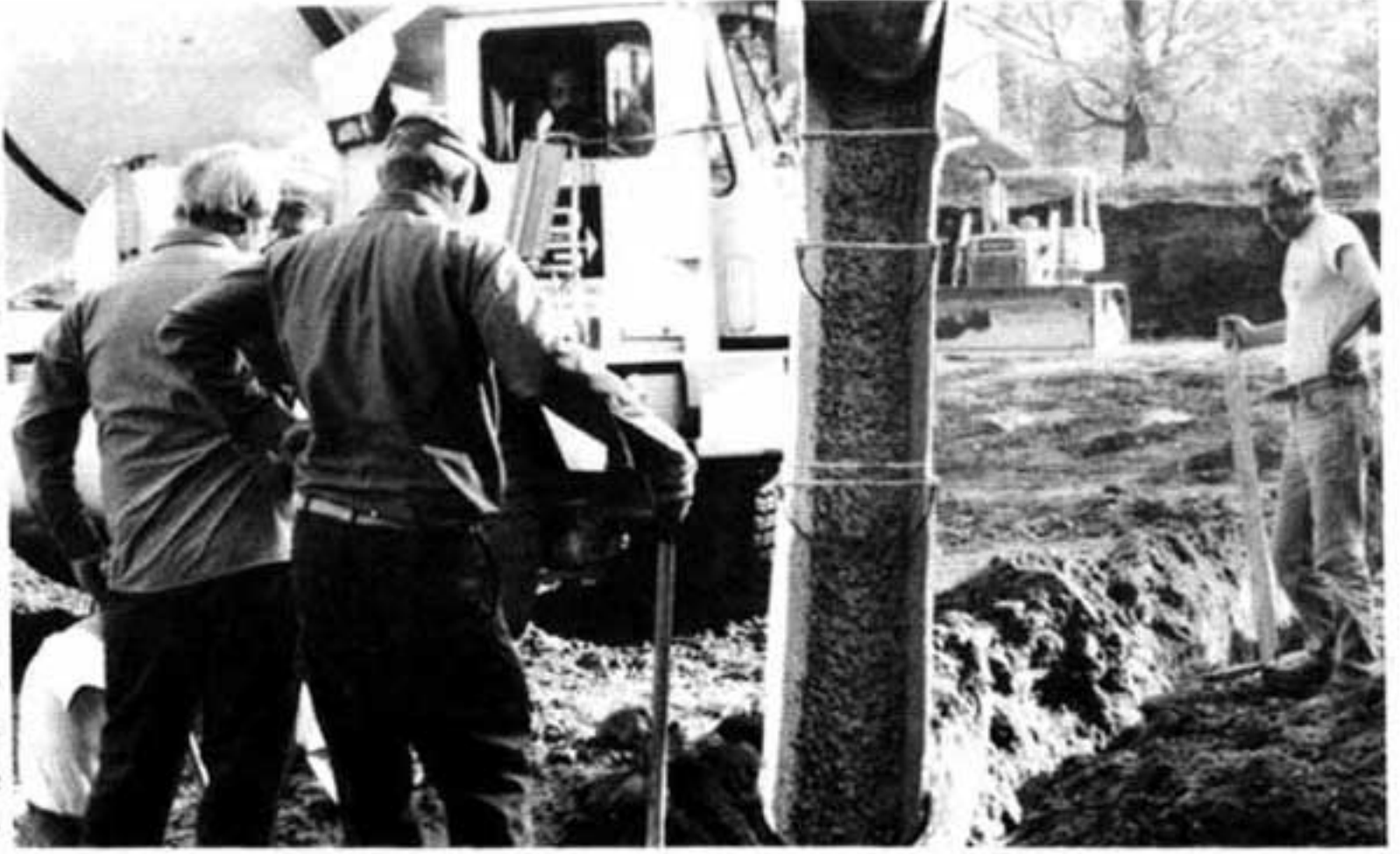
READY... AIM... FIRE! Workmen direct the pouring of the concrete footings for the new seminary chapel.
